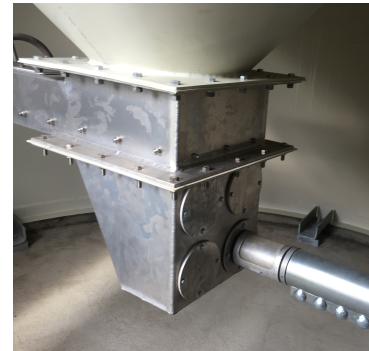
Silo Outlet with Slide Gate and Vacuum Take-off Box
