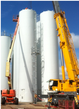
Full Installation Services
